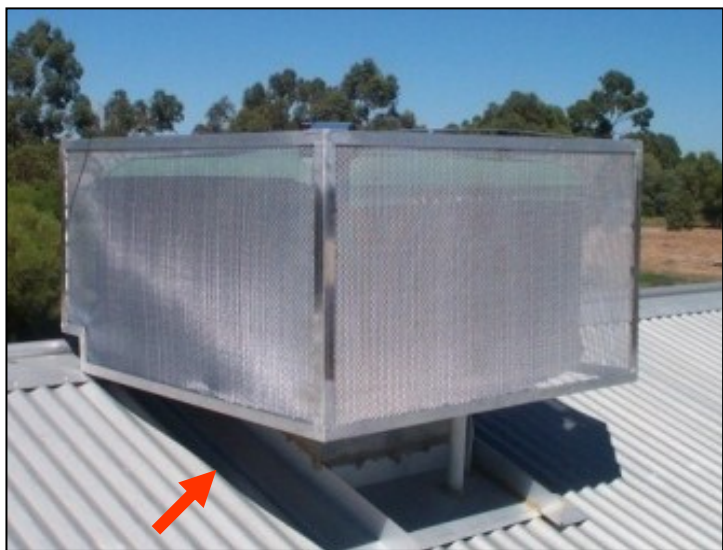
Figure 4. The unit cover pictured does not enclose the bottom of the air conditioner and therefore does not adequately protect it from ember attack.
