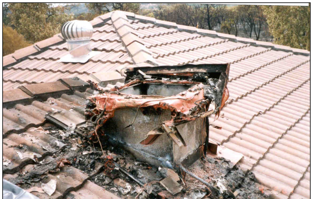
Figure 1. An evaporative air conditioning unit burnt during a bushfire.
