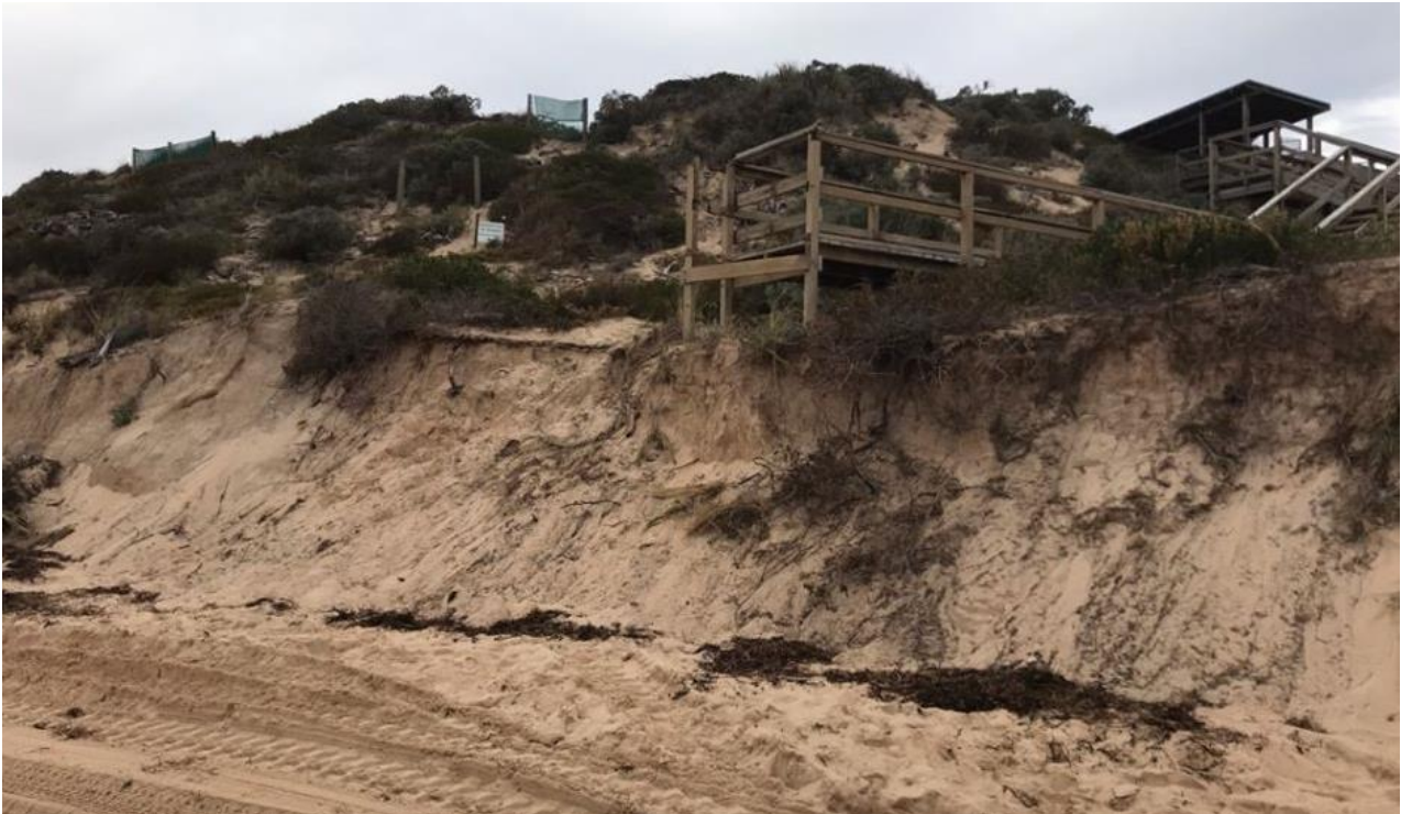
FIGURE 4-10 DALYELLUP BEACH ACCESS STAIRS DAMAGED IN WINTER 2020 STORMS (COASTSNAPWA VIA UWA, 2020).
