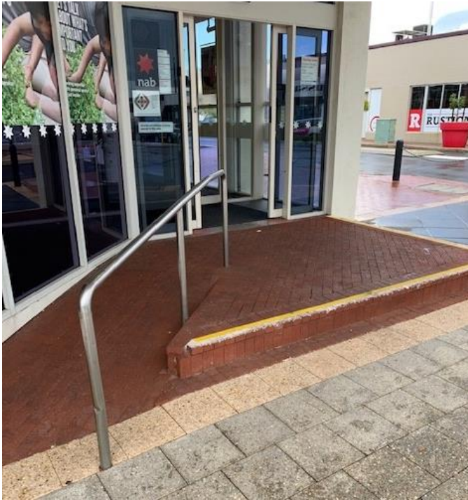
Above: A bank with an unacceptable stepped entry point.
